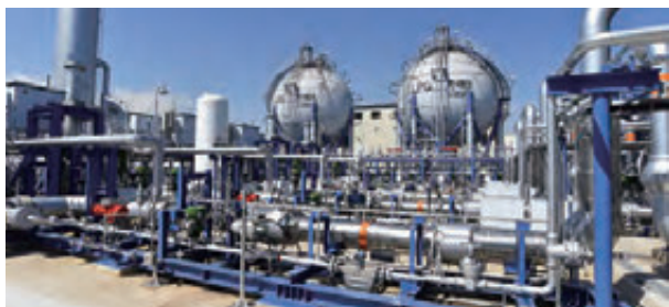
Calorific value adjustment system at Ogishima Natural Gas Supply Co., Ltd.
