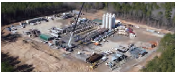
Shale gas mining area of Sabine Oil & Gas Corporation in the United States
