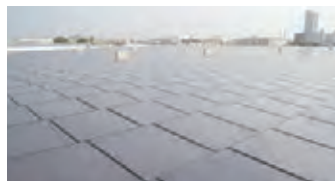
Torishima Solar Power Plant
