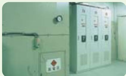
Inverter control room (Panjo Shopping Center)
