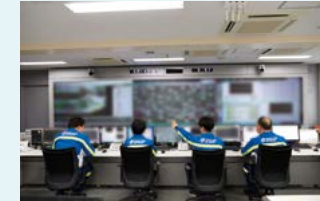
Central Control Room
