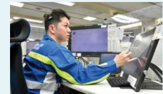
Central Control Room (emergency call reception)
