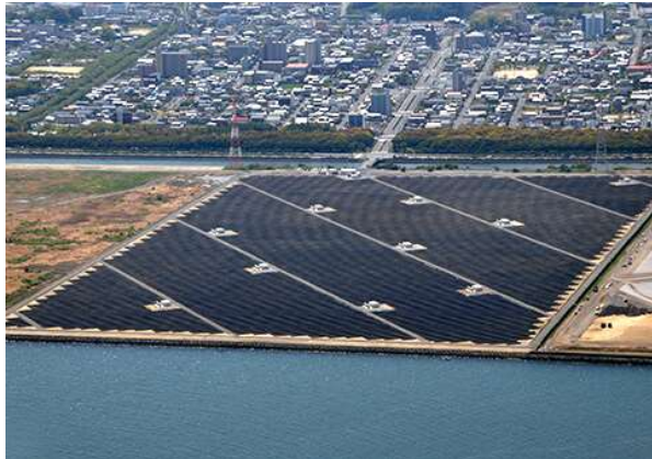
Figure-2 Daigas Oita Mirai Solar Power Plant
