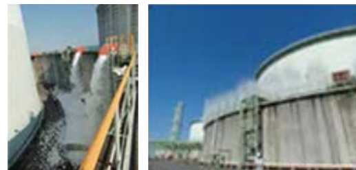
High-expansion foam discharge and water curtain facilities along the dike around an LNG tank
